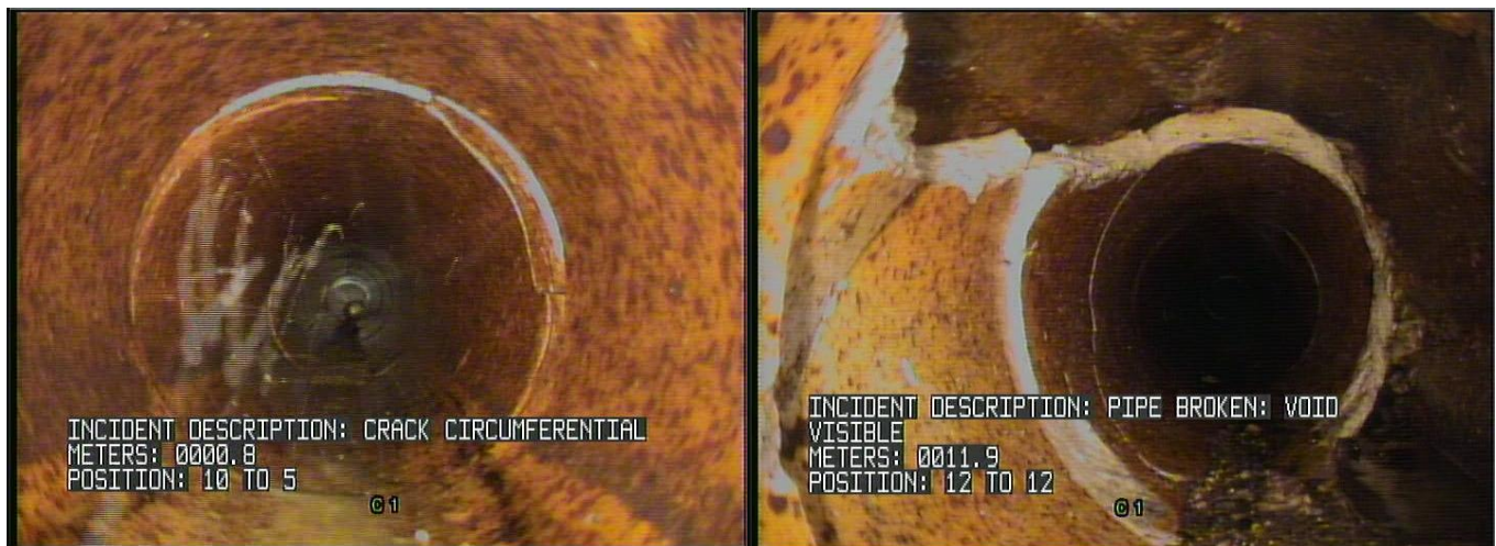
Figure 27 - Structural Condition Trigger for Pipe Bursting (Replacement) on Sanitary Pipe #JSD023
