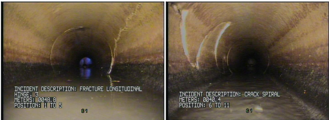
Figure 26 - Structural Condition Trigger for CIPP on Sanitary Pipe #JSD012
