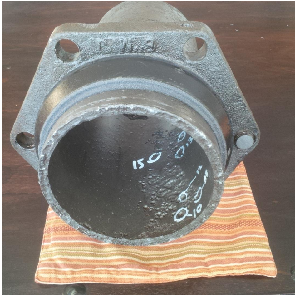
Figure 4 – Jasper Water Main #2871
