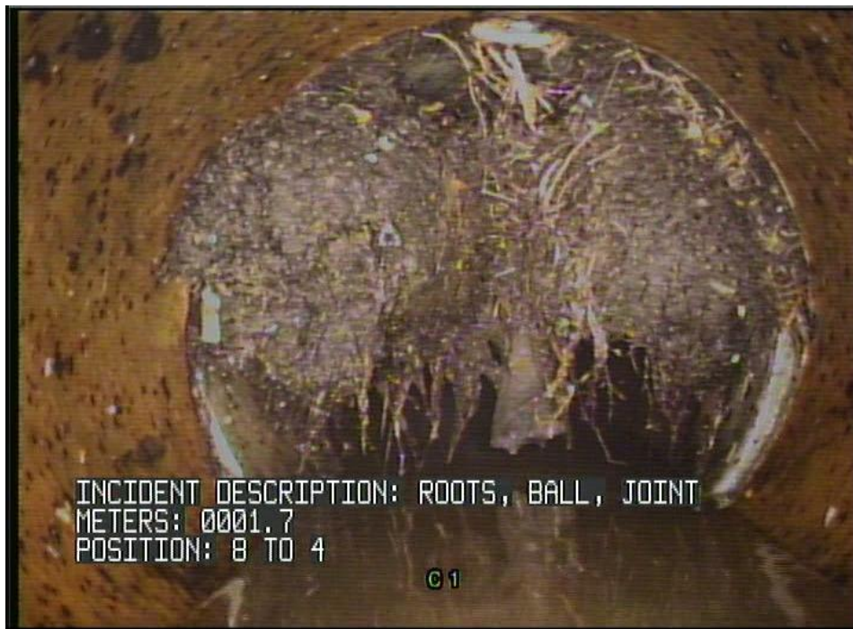
Figure 25 - O&M Trigger for Sanitary Pipe #JSD039
