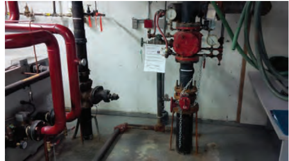
Activity center incoming water services
