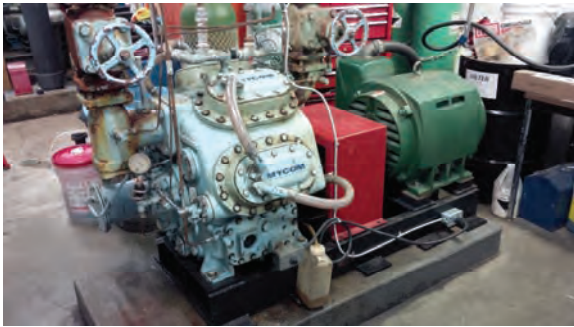
Refrigeration plant reciprocating compressor
