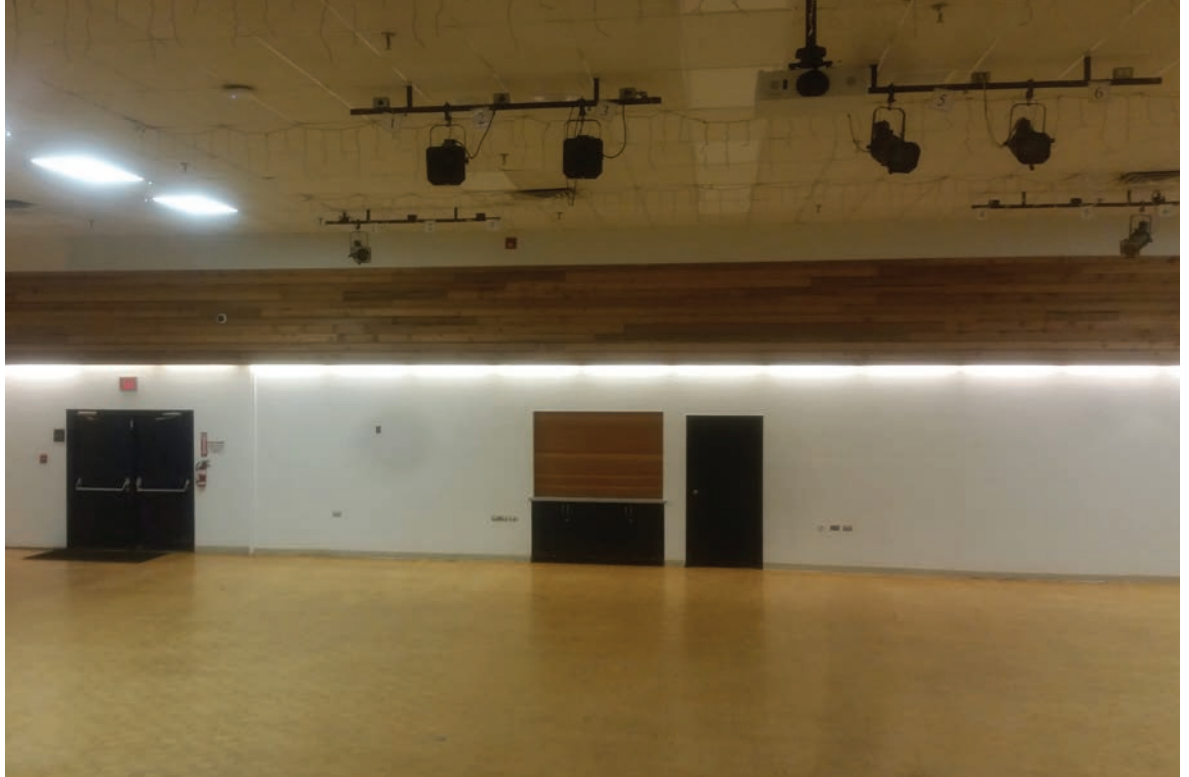
Image 3, Multipurpose room finishes. Ceiling tiles are worn, wall finishes are dated and floor is past it's serviceable life span
