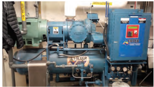
Refrigeration plant screw compressor
