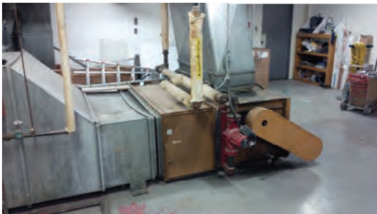
Activity center basement AHU
