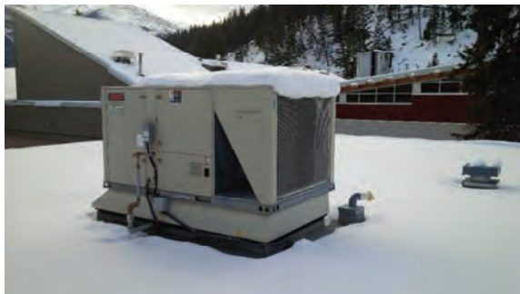
Typical roof-top heat/cool unit
