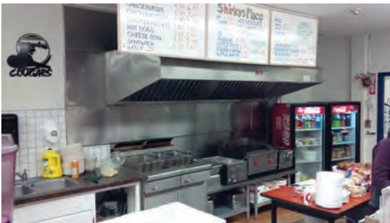
Kitchen exhaust hood
