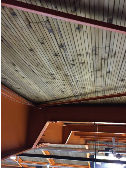
Figure 5.1: Arena – Steel Roof Structure (Water Staining of Timber Decking)
