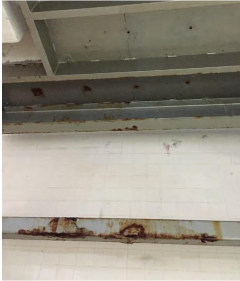
Figure 5.5: Natatorium – Steel Stair (Corrosion of Typical Stair Members)
