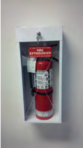
Typical wall mounted FEC
