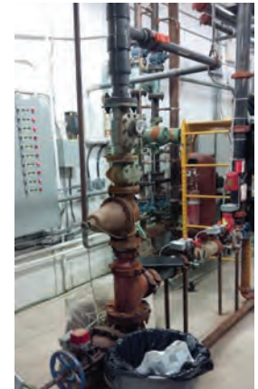
Aquatic facility incoming water service
