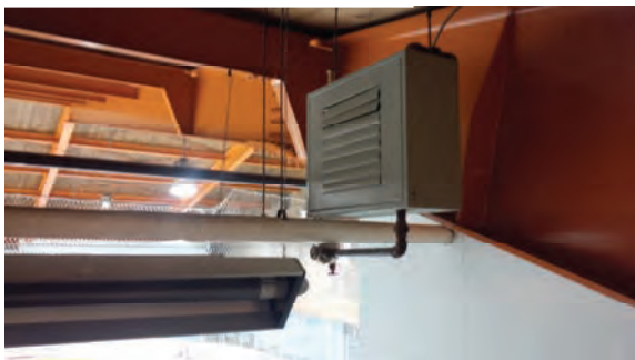
Redundant hot water unit heaters in arena
