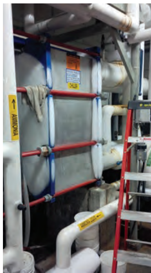
Refrigeration plant plate & frame chiller
