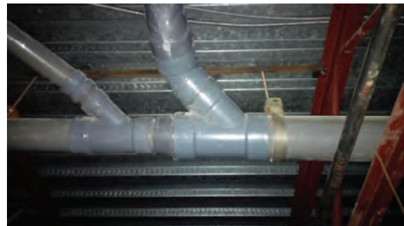
Plastic pipe in basement R/A plenum
