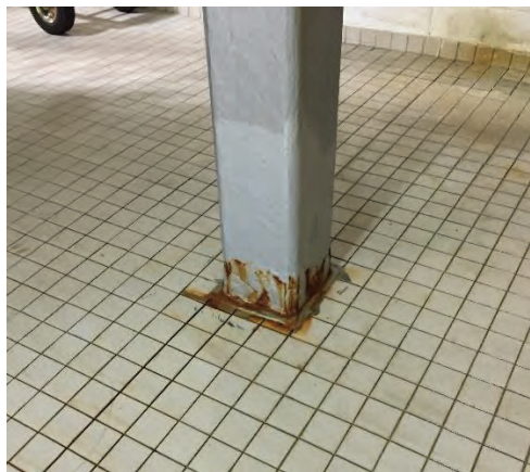
Figure 5.4: Natatorium – Main Floor Column (Corrosion at Base of Columns)
