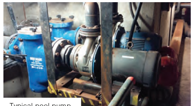
Typical pool pump
