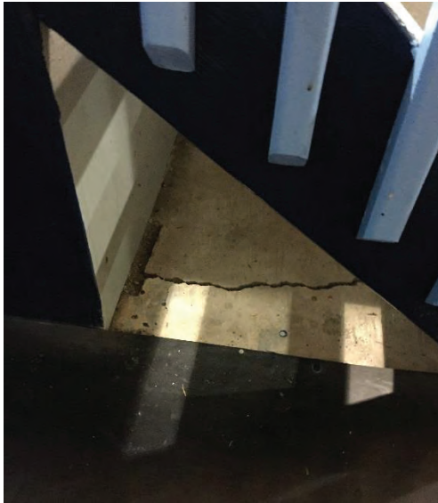
Figure 5.2: Arena – Main Floor (Slab-on-Grade Crack)
