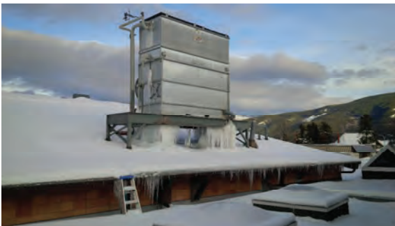
Refrigeration Plant Roof mounted condenser
