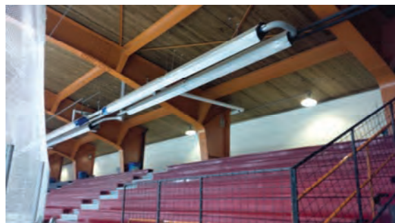
Arena infrared heaters
