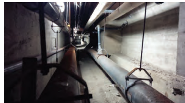
Pool piping in tunnel
