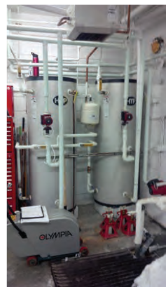
Arena flood room hot water heating
