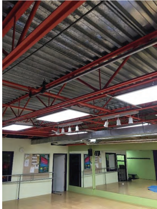
Figure 5.3: Multi-Purpose Hall – Main Floor Steel Structure (Missing Fire Spray)
