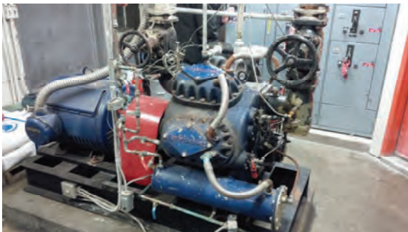
Refrigeration plant reciprocating compressor
